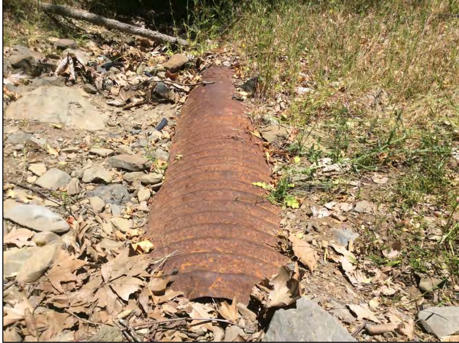
Photo 5. Nonfunctional culvert at SC3.
