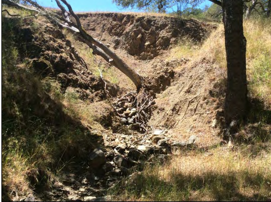
Photo 1. A large gully near stream crossing SC1, downstream of the road.
