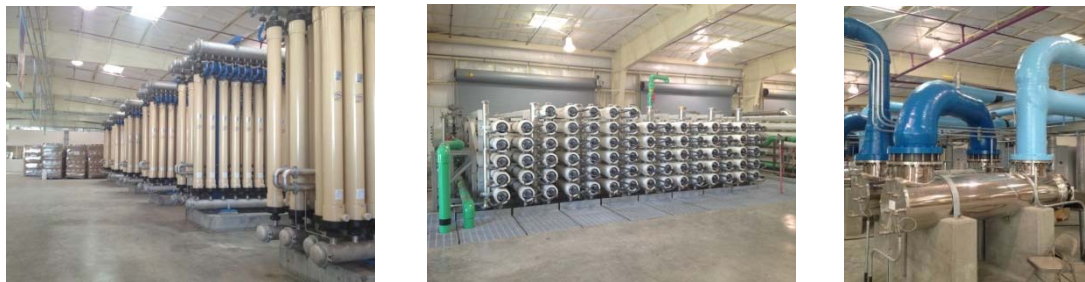
Figure ES-5 SVAWPC Full-Scale Advanced Treatment Processes
