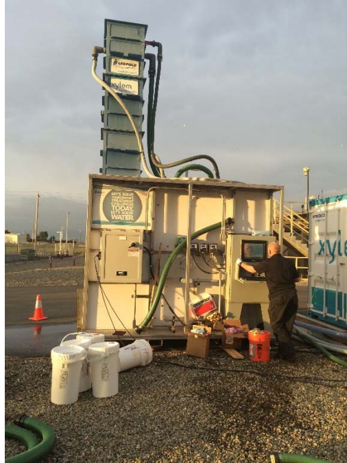
Figure 6.11 Leopold Biofiltration skid next to the Xylem advanced oxidation pilot at the District.
