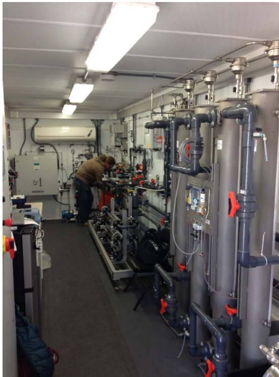
Figure 6.10 Interior of the Xylem Mipro advanced oxidation pilot system trailer on-site at the District
