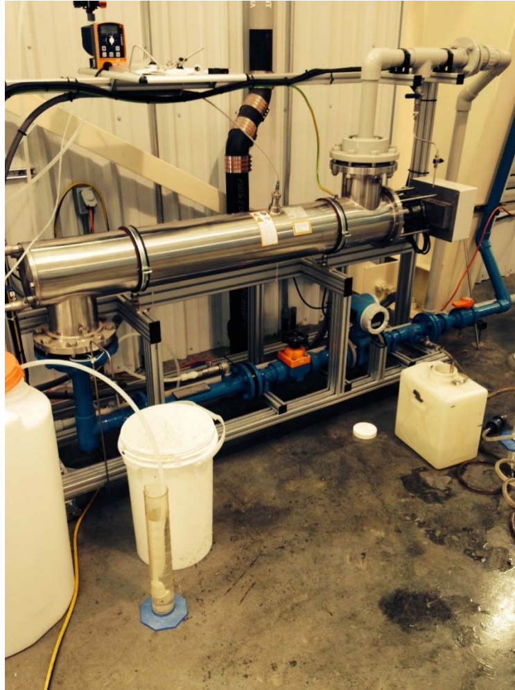
Figure 5.1 Xylem LBX90 reactor during testing at the SVAWP
