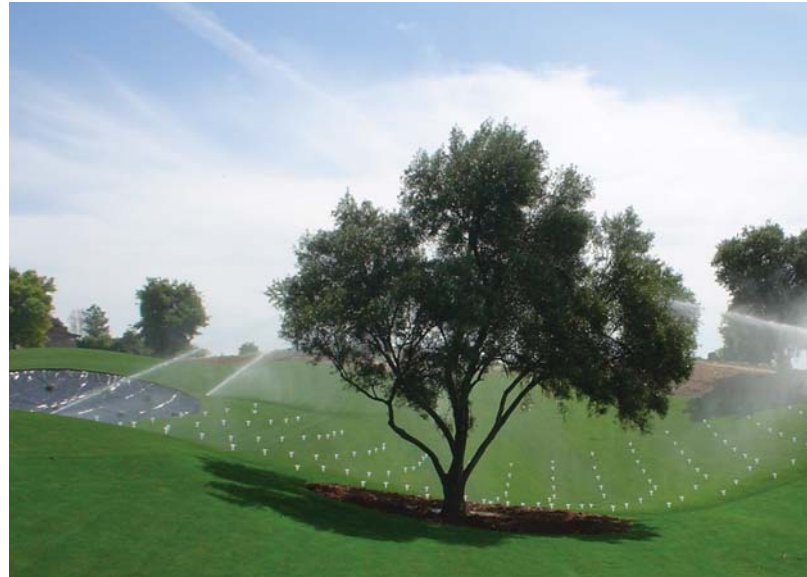
Irrigation system evaluation at a golf course in Morgan Hill.
