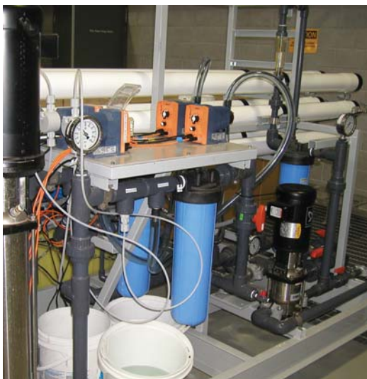
Pilot apparatus set-up at Alameda County Water District.
