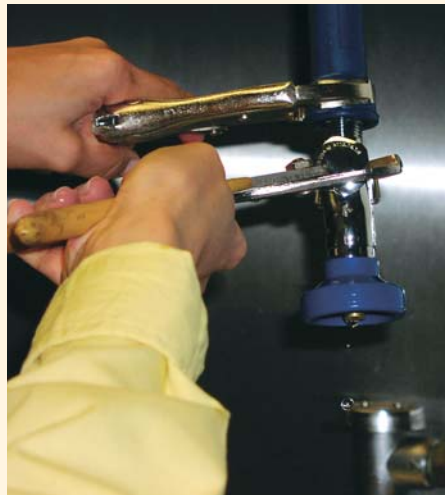
Installation of a new high efficiency spray valve under the Rinse & Save program.
