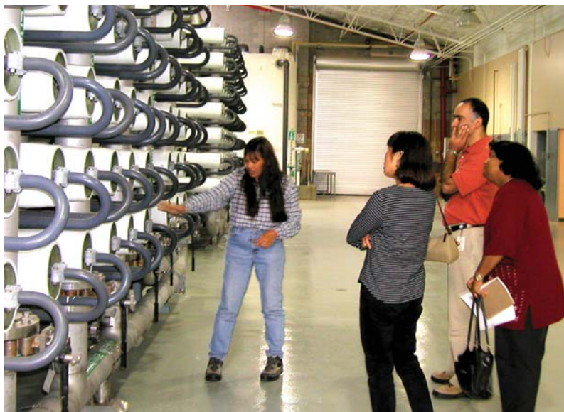
Educational tour of 5-mgd brackish water facility (full-scale) at Alameda County Water District.
