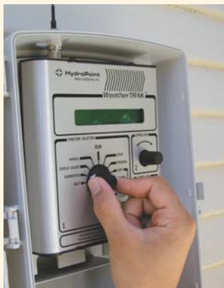
Setting an ET irrigation controller.
