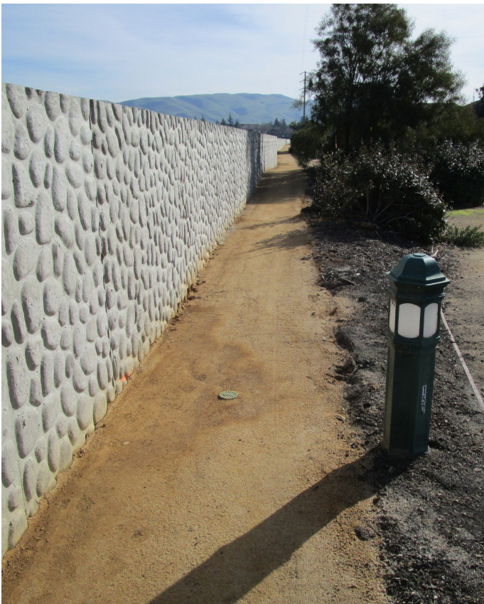
A completed floodwall section, located between N. Hillview Dr. and N. Milpitas Blvd.
