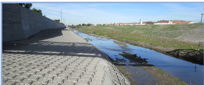
Completed Lower Berryessa Creek flood improvements between North Milpitas and Calaveras boulevards.
