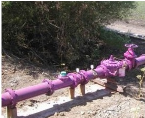
Non-potable reuse (purple pipe) reduce demands on potable supplies.
