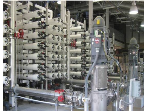
Reverse osmosis is one step in the advanced treatment process for purified wastewater
