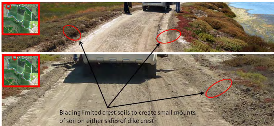
Figure 6 – Blading and scarifying dike crest silt to either side of the crest – to create limited crest elevation rise.
