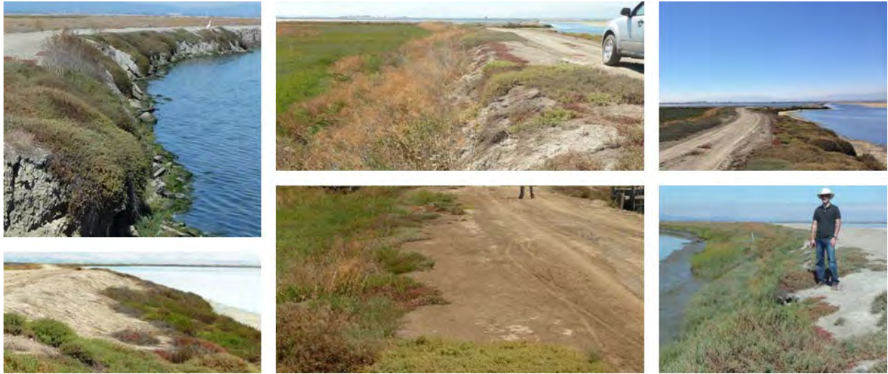
Figure 15 - Vegetation is covering much but not all the dike slopes
