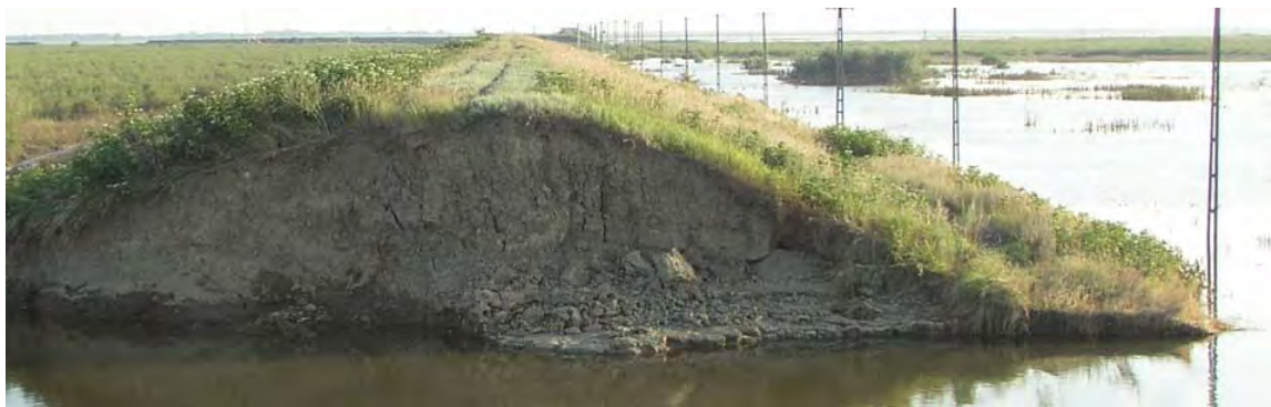
Figure 13 - Failed levee in Romania due to rodent tunneling holes
