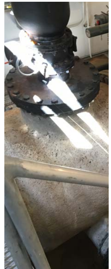
Shannon line valve
