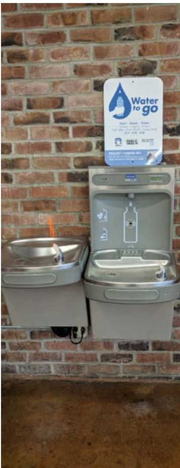
Fremont High School Water to Go - a filling station funded by the 2012 Safe, Clean Water Program
