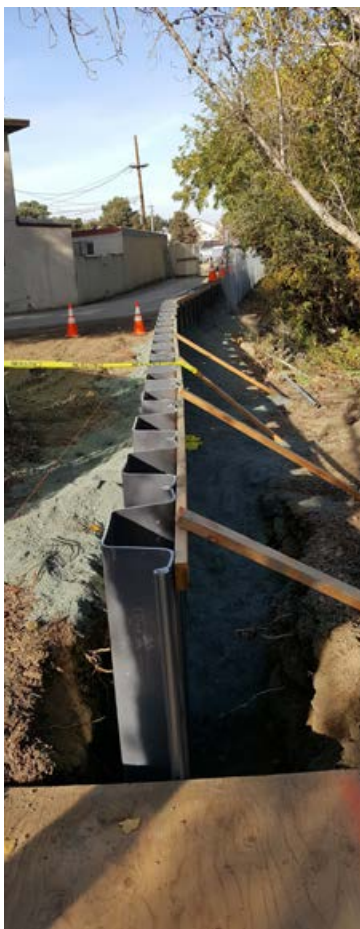
Interim floodwall and embankment along Coyote Creek in the Rock Springs community
