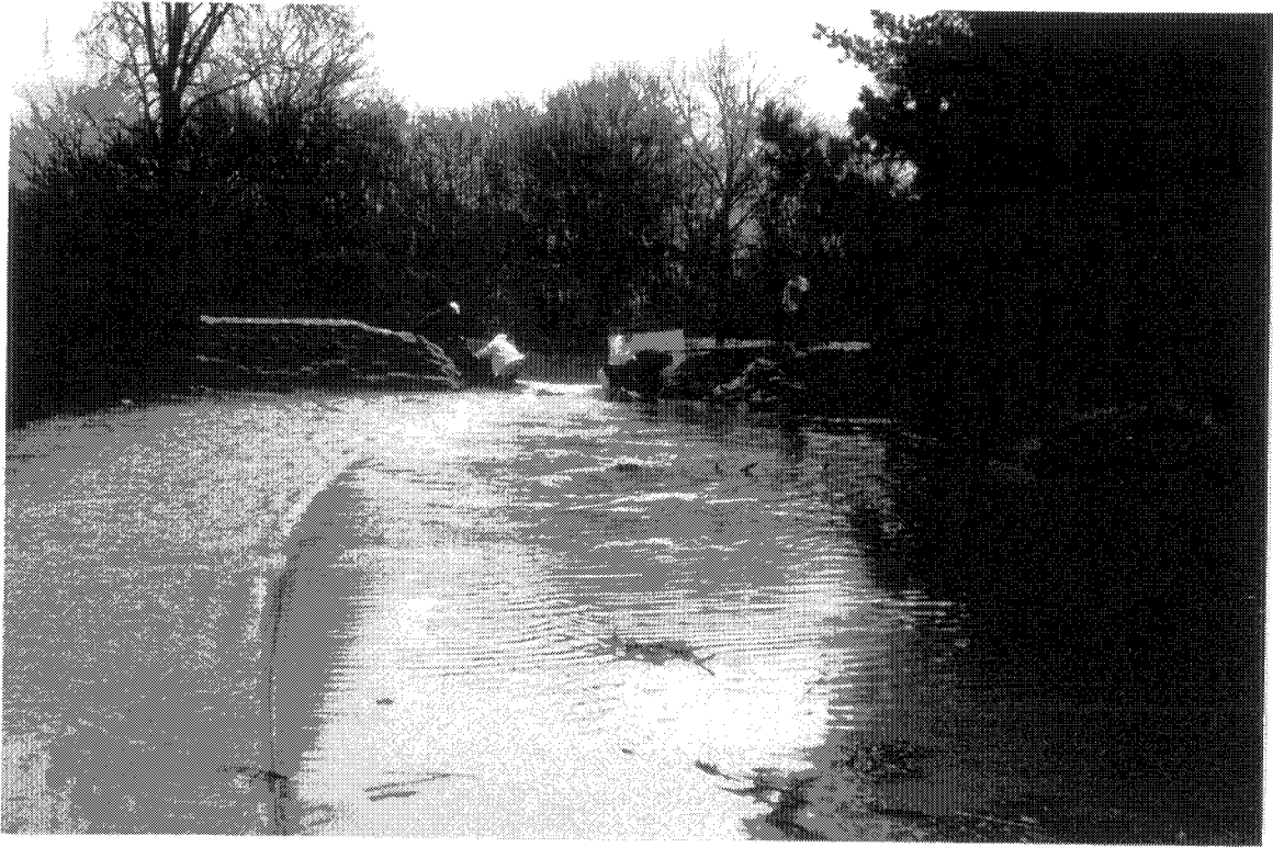
Coyote Creek in San Jose - Water District crew building sandbag levee at railroad crossing to protect mobile homes 1-26-97 (S5074-18)
