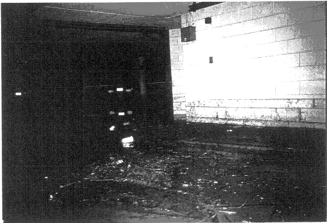
High water mark and debris in underground garage from San Francisquito Creek flood waters (Palo Alto) 2-3-98 (S5199-15)
