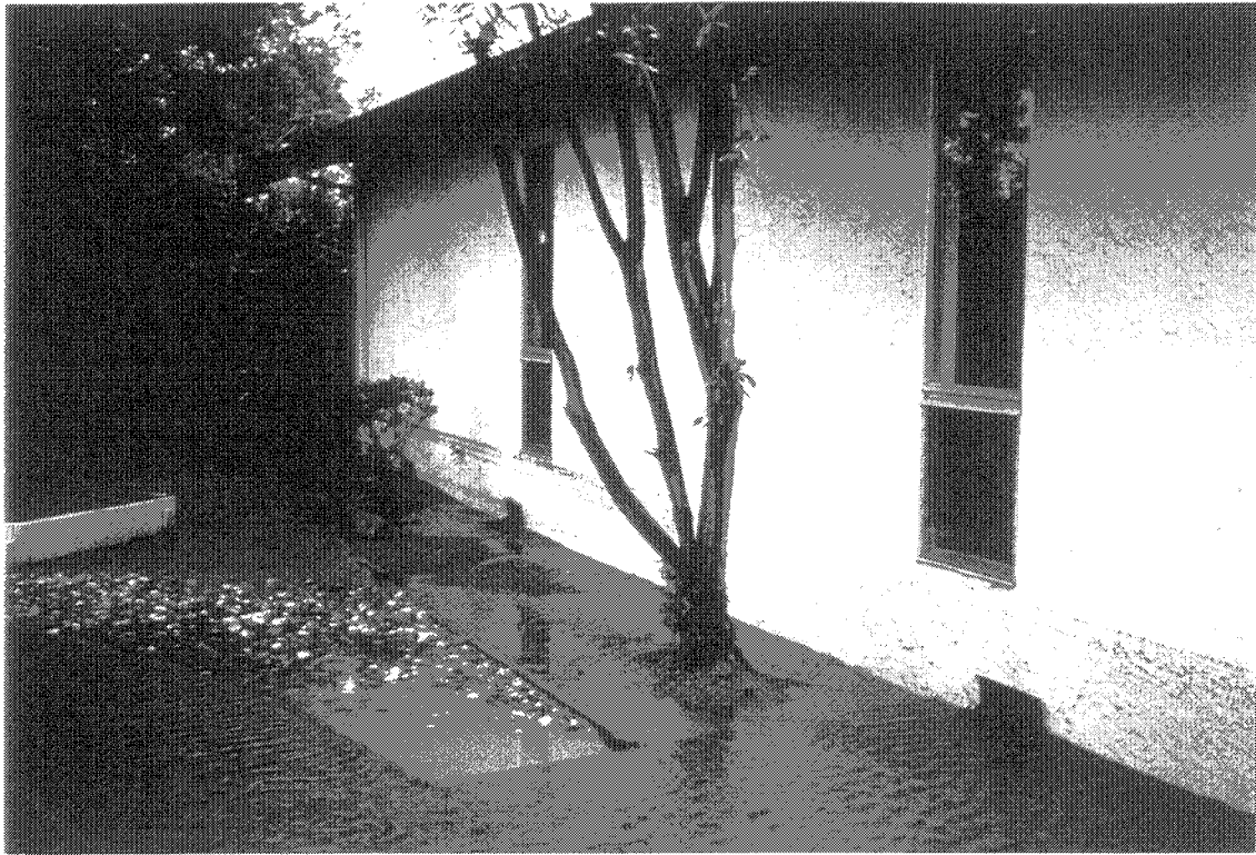
High water mark from Calabzas Creek flooding on home located on Miller Avenue in Cupertino 2-3-98 (S5255-1)
