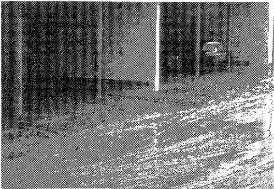
Mud deposited in parking garage of Fountainbleu Apartments on Miller Avenue in Cupertino by flood waters from Calabazas Creek 2-8-98 (S5215-11)
