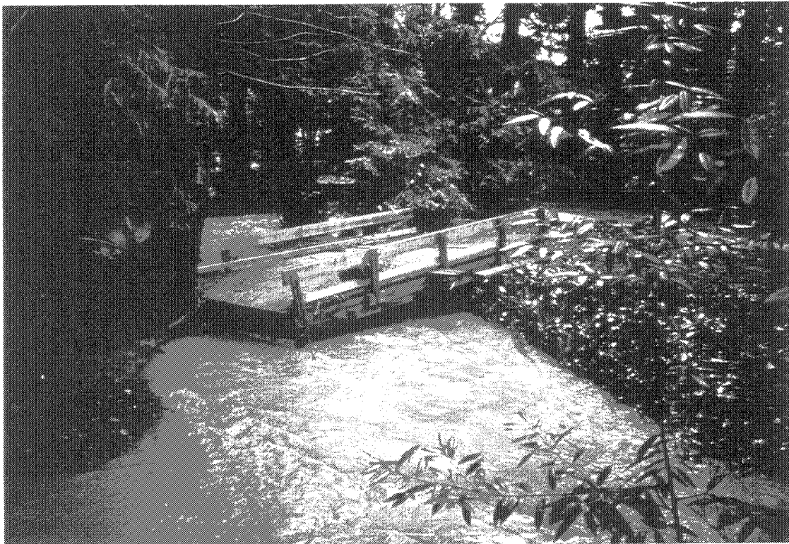
Bridge torn from moorings by Adobe Creek flood waters Los Altos Redwood Preserve 2-4-98 (S5255-19)
