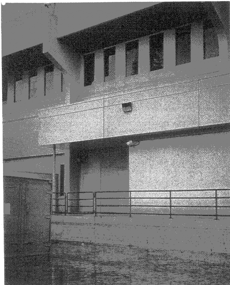
High water mark from Calabazas Creek flood waters on loading dock of Tandem Computers on Tantau Avenue in Cupertino
