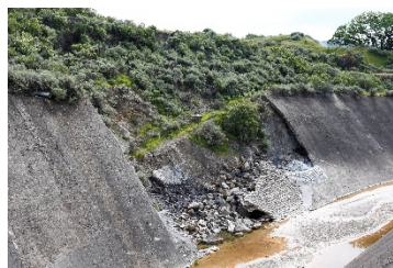
Damaged spillway of existing North Fork Dam
