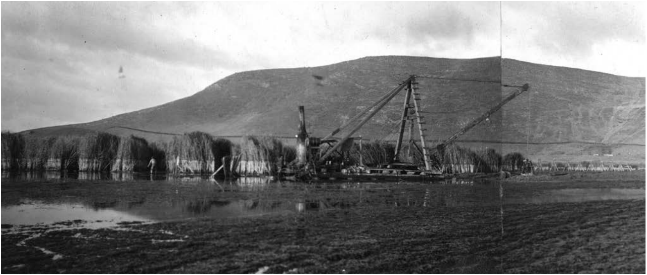
FIGURE II-11. "LAGUNA SECA RECLAMATION", 1916. "Bottom of Lagoon on December 28, 1916, showing Clam-shell machine at end of Ditch. Discoloration on tules [sic] shows height of water before drainage. Small shallow pools are from drainage water still coming from tules and flowing to Ditch" [text from original photo caption] (SCVWD Vault 1916: 66-67).
