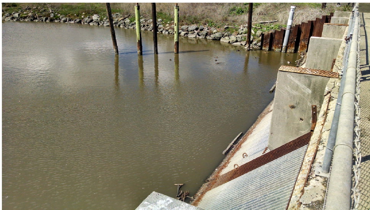
Figure 30. PAFB Tide Gate Condition
