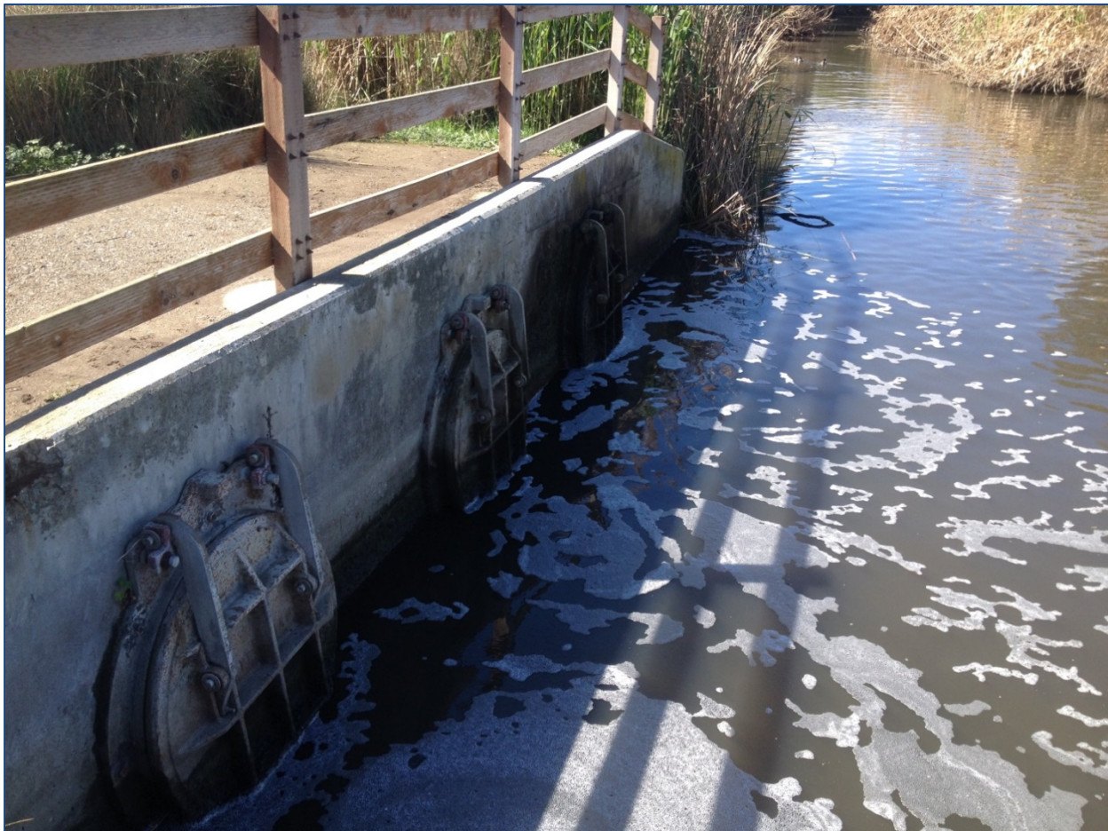
Figure 10. Coast Casey Pump Station Outfall to PAFB
