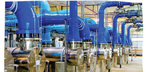
#3 UV LIGHT DISINFECTION AND ADVANCED OXIDATION
