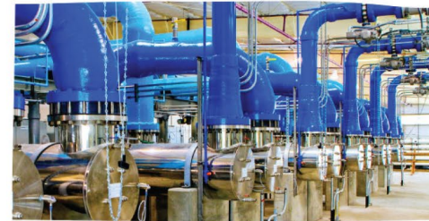
#3 UV LIGHT DISINFECTION AND ADVANCED OXIDATION
