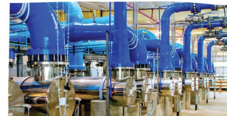
#3 UV LIGHT DISINFECTION AND ADVANCED OXIDATION
