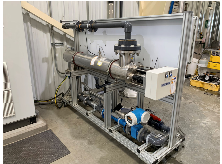
Upgraded UV/AOP system at SVAWPC
