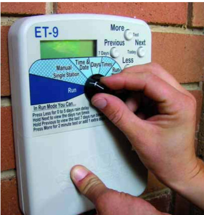
Adjusting the controller of a residential water-efficient landscape irrigation system.
