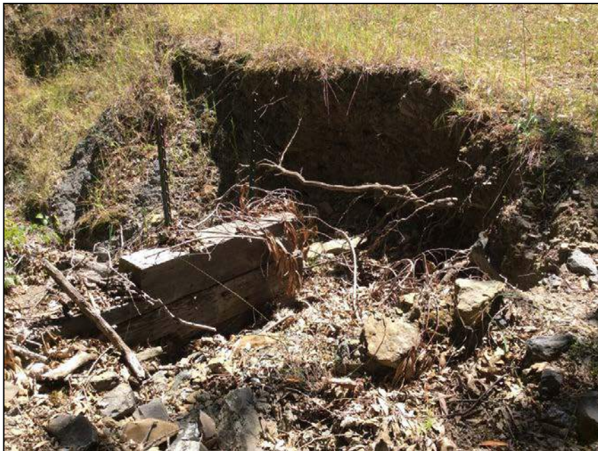
Photo 2. Damaged wooden retaining wall and headcut at SC4, just downstream of the drivable road. This stream is ephemeral and only conveys flows during and immediately following storm events.
