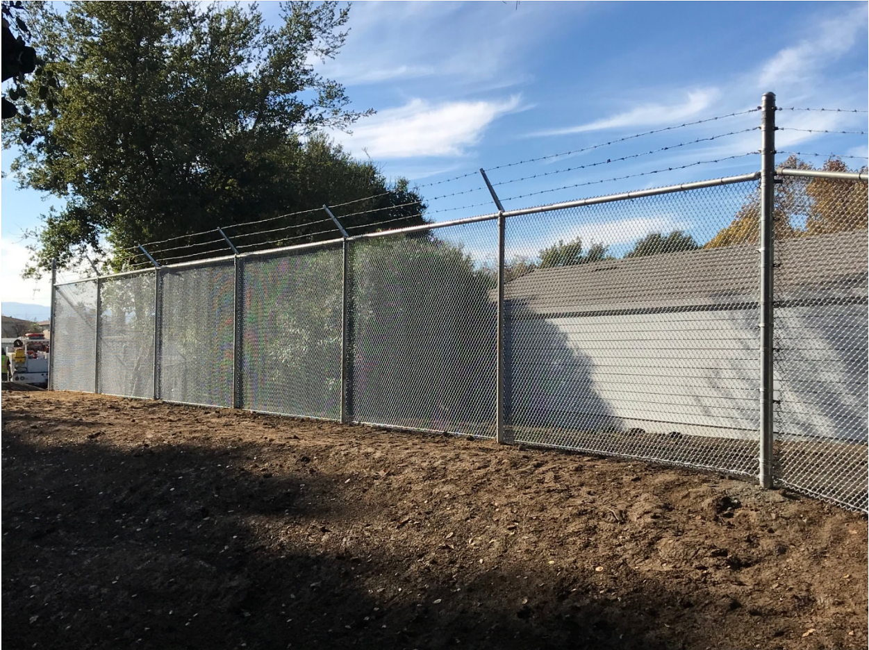
1" Galvanized fence fabric (barbed wire on top not typical)
