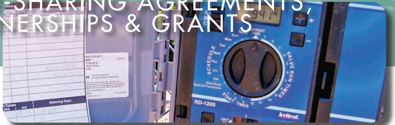
Irrigation controller at local residence.
