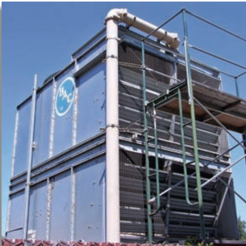
Valley Water offers a rebate on cooling tower conductivity controllers.
