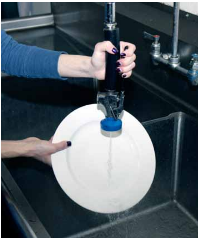
A high-efficiency pre-rinse spray valve in use.
