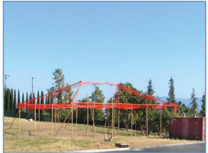
The maintenance building will occupy a flat area on the plant's south-east section. Poles show the building's approximate dimensions.
