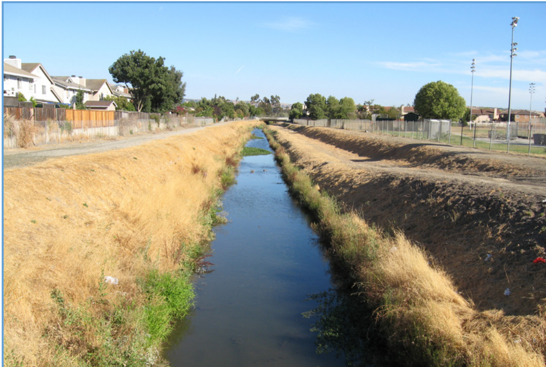
Existing: Looking upstream from Ocala Avenue; limited carrying capacity and noticeable bank erosion.
