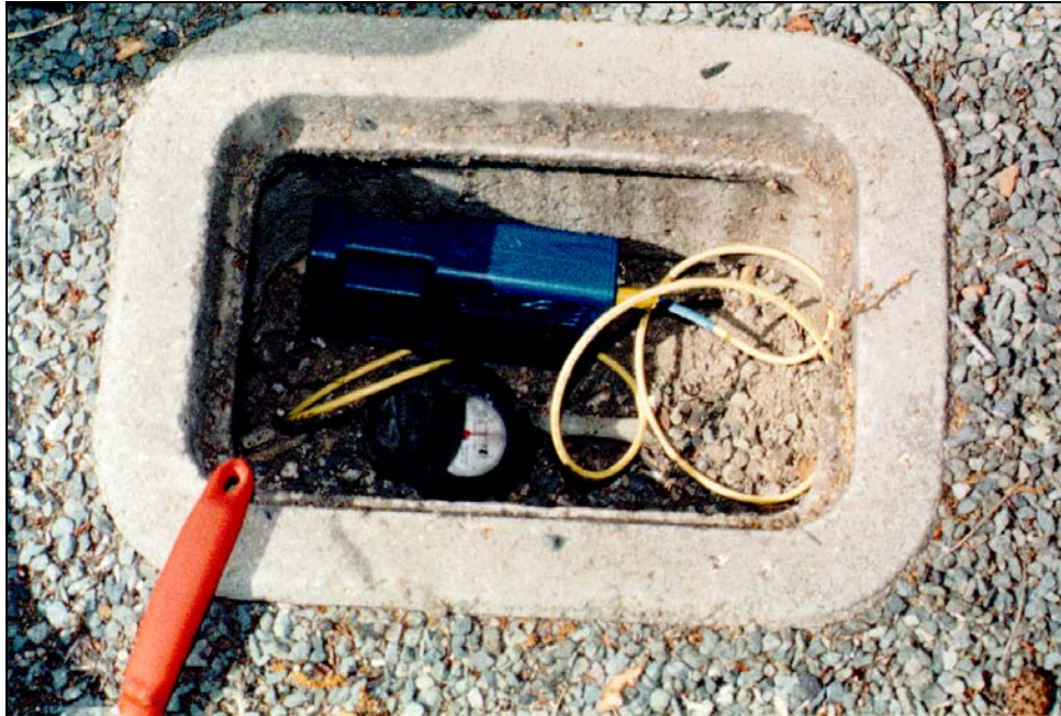
Figure 2: Example of a data logger installed on a residential meter (photo supplied by Aquacraft, Inc.)
