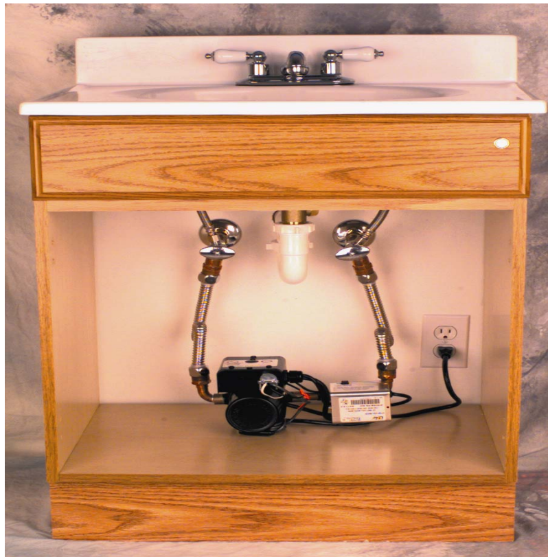
Figure 1: Example of a hot water re-circulation device installed under a sink (photo supplied by ACT, Inc. Metlund Systems)
