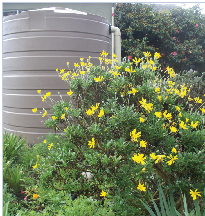
A well designed rainwater harvesting system, 865 gallon cistern in a residential backyard. (Photo credit: Ecology Action)
