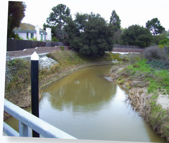
A debris deflector protrudes up from beneath the Bayshore Freeway bridge, where it prevents the accumulation of flood debris that can block water flow and cause flooding to nearby homes. The facing page photo shows debris accumulating at this same bridge before the deflector was installed.
