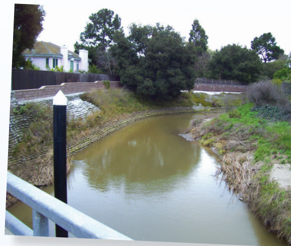
A debris deflector protrudes up from beneath the Bayshore Freeway bridge, where it prevents the accumulation of flood debris that can block water flow and cause flooding to nearby homes. The facing page photo shows debris accumulating at this same bridge before the deflector was installed.
