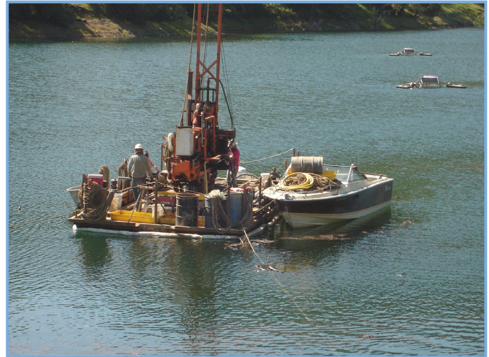
Soil samples are obtained at Almaden Reservoir using a drill rig mounted on a barge.
