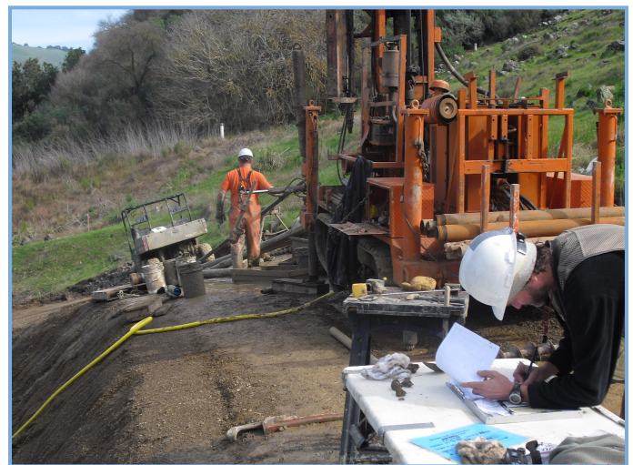
Soil samples are obtained on Calero Dam using a mud rotary drill rig mounted on tracks.
