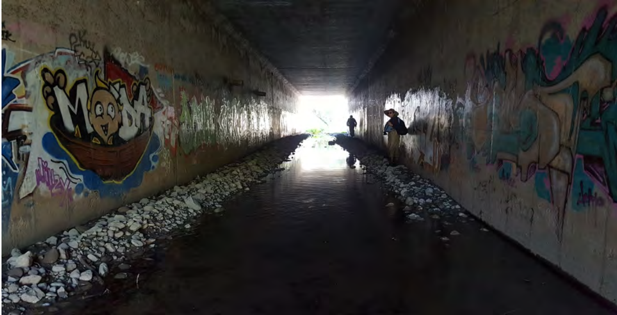
Culvert 1: Primary passage culvert, looking downstream. Note low-flow channel shape provides suitable depth.
