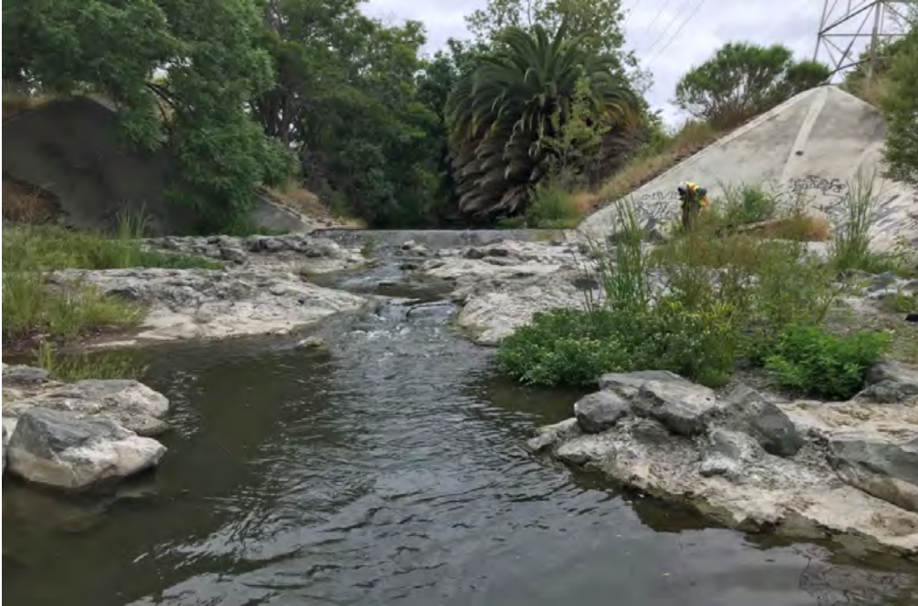
View from downstream looking upstream at grouted rock veins and concrete drop structure
