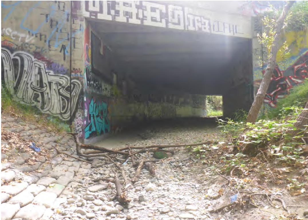
Culvert outlet, looking upstream with some concrete exposure on outside of bend
