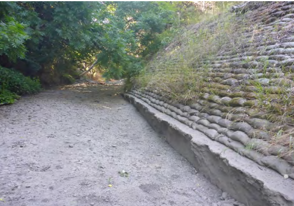
Right bank sacrete revetment with undermined toe, looking downstream from grouted boulders
