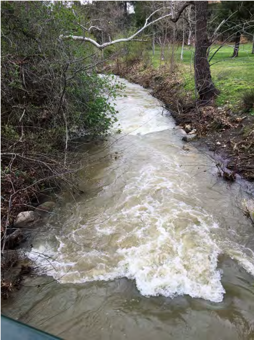
Photograph 2. Potential fish passage impediment downstream of footbridge.
