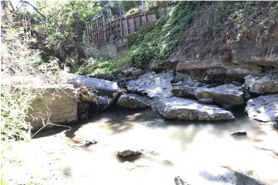
Looking upstream at concrete rubble across channel located downstream of the crossing
