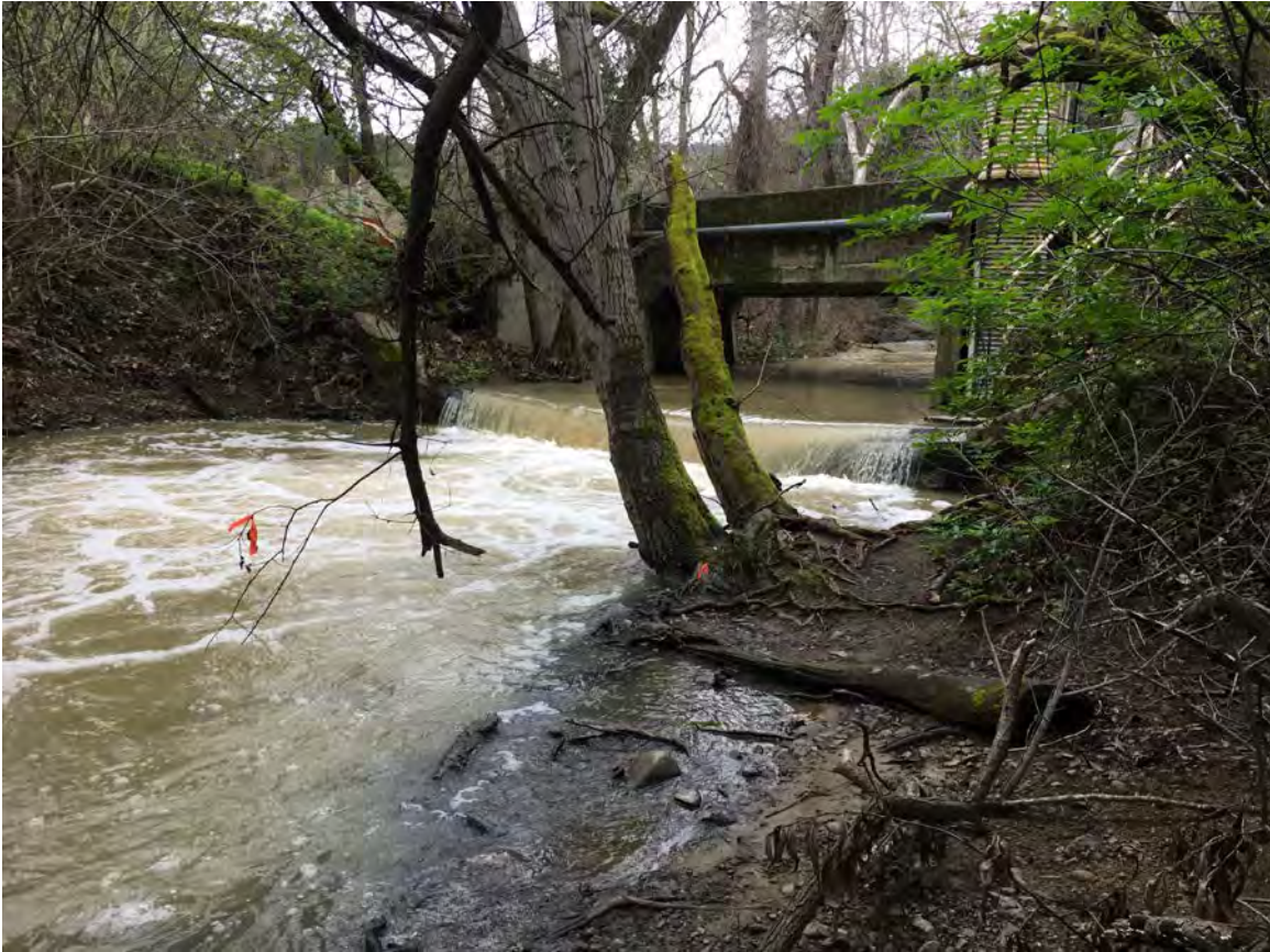
Photograph 1: Potential fish passage impediment at gauge weir at Stevens Creek Park
